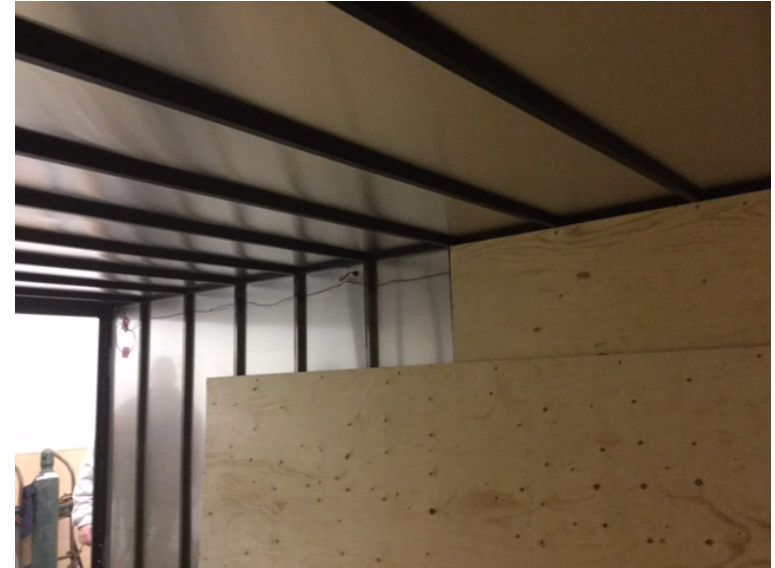
16 inch centres and rubber coated frame work
